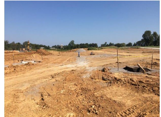
Storm Lines & Sprinkler
