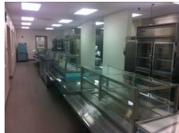
New Kitchen Serving Line
