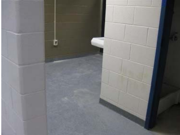
Epoxy Flooring in Restrooms
