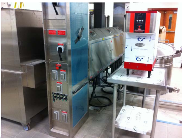
Utility Distribution System
