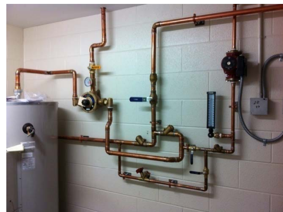
Plumbing Piping & Gages
