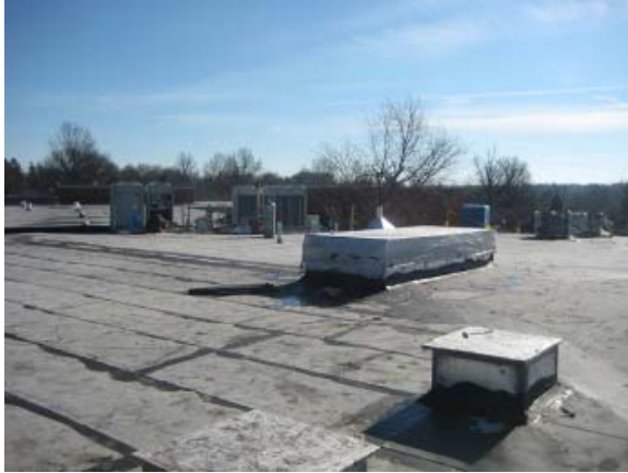
Roof w/ New Mechanical Units
