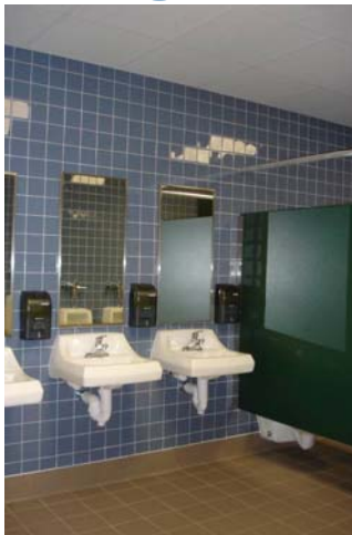
New Gang Restrooms
