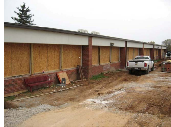
Classroom Windows Awaiting New Windows
