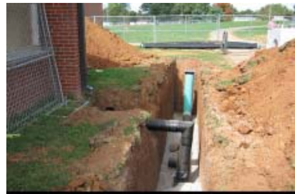
Storm Water Management
