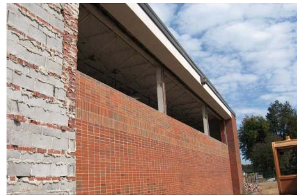
Gym Window Structural Support
