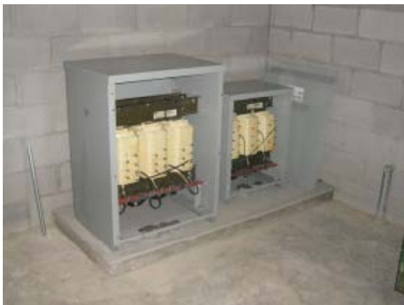
New Electrical Equipment
