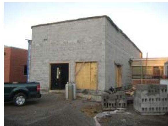
New Mechanical Room
