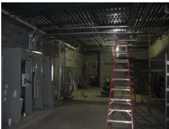
Mechanical Room with Switch Gear
