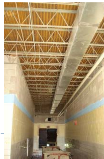
New HVAC Ductwork
