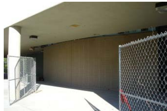
New Electrical Room
