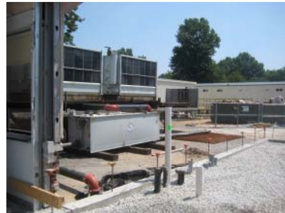
Temporary Chiller Location
