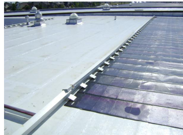
Solar PV Panels on Roof
