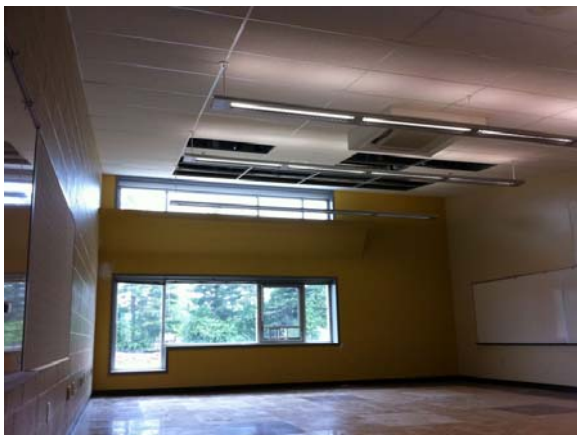
Lights in South Classrooms
