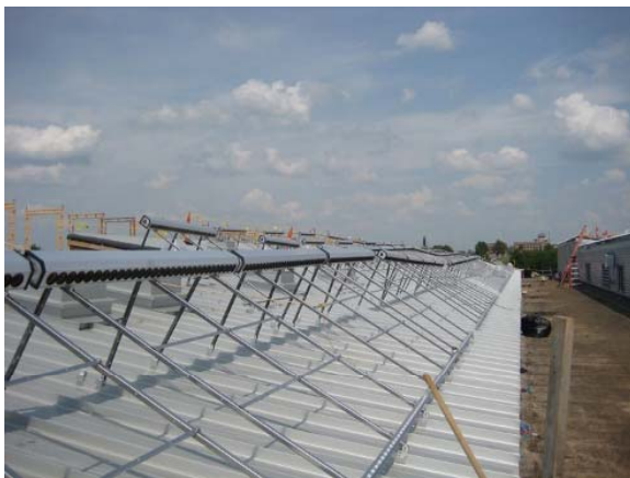
Roof w/ Solar Thermal Heating Tubes
