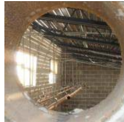
Academic Bldg. – Overhead Piping in Lab
