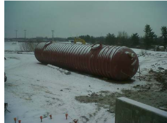
Rainwater Collection Tank
