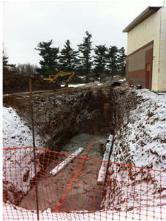
Rainwater Collection Tank
