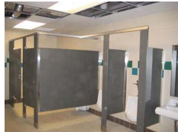
Tile in Boys' Restroom
