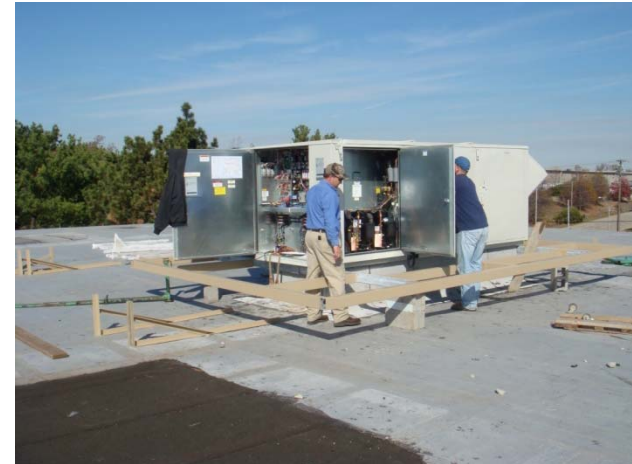
Gym Make-up Air Unit
