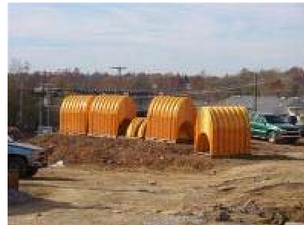
Underground Retention System
